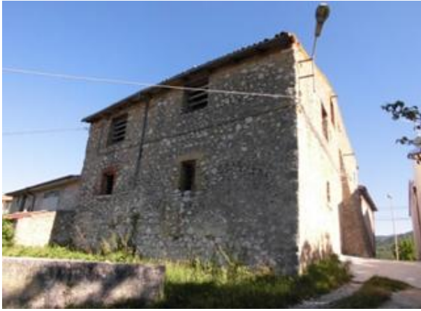
Figure 3. Typical historic building in Alzano made by sandstone blocks. This building was affected by the earthquakes of 1703 and 1915, whose effects are still apparent today.
